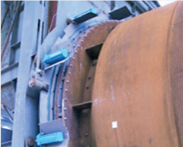
Inlet to the rotary kiln
