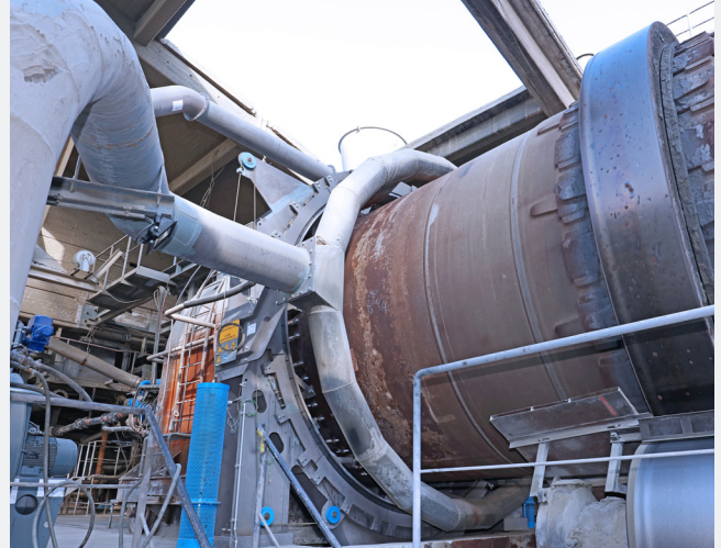
Graphite seal at a rotary kiln on the kiln outlet side.
