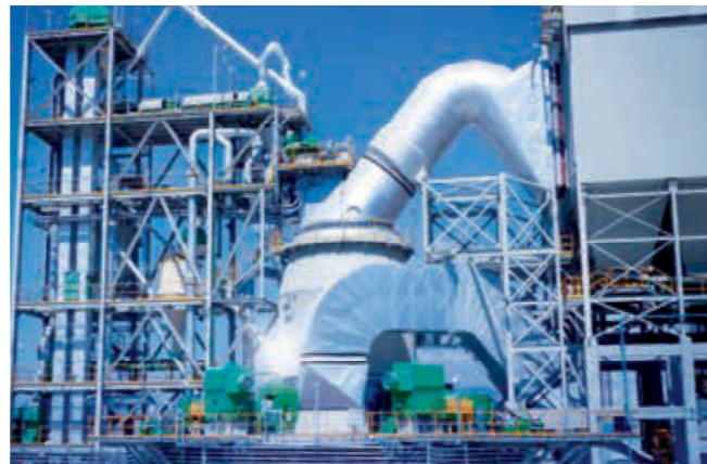
The largest QMC 2 -RD is installed in Mexico. The system has a rating of 4 x 1,800 kilowatt and a capacity of 300 tonnes per hour.
